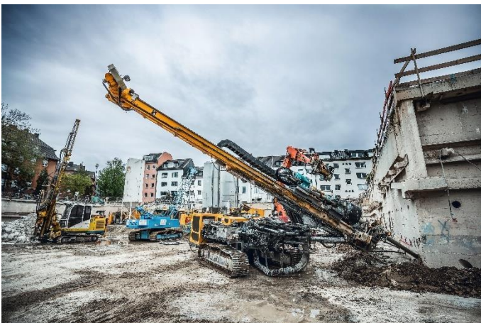
(2) Powerful equipment from Bauer Maschinen, KLEMM (pictured) and RTG are in use for the specialist foundation engineering work.
