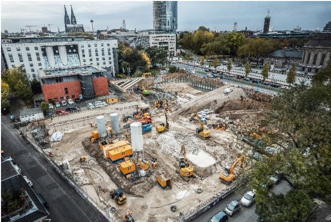
(1) Bauer Spezialtiefbau constructs a complex 8 m deep excavation pit for the new LVR building at Ottoplatz in Cologne.
